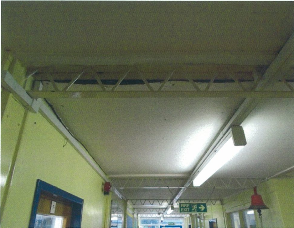
Photo 13 Failing Ceiling Boards
