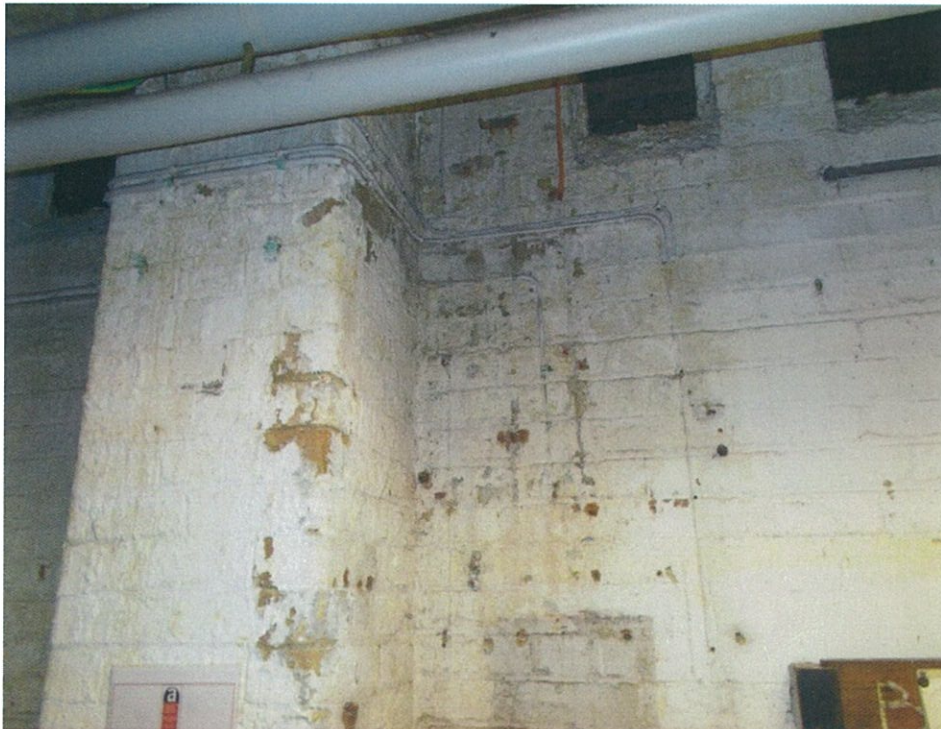
Photo 18 Water Ingress into Basement
