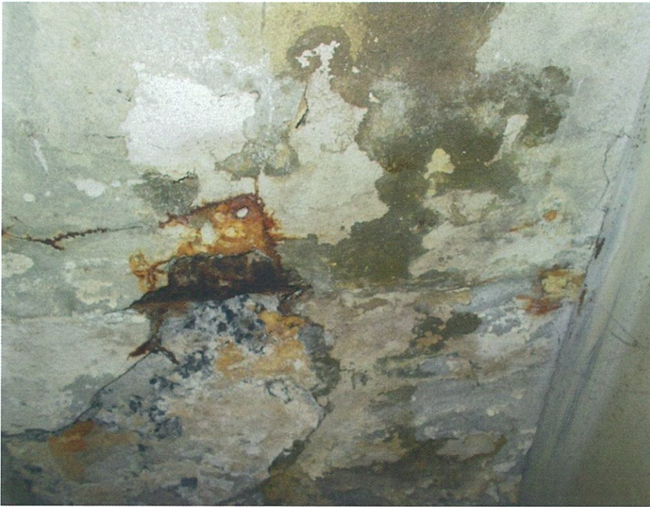
Photo 17 Corrosion to Embedded Steel within Basement Ceiling
