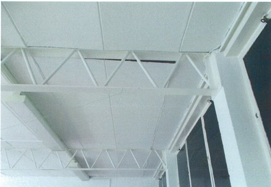
Photo 14 Failing Ceiling Boards
