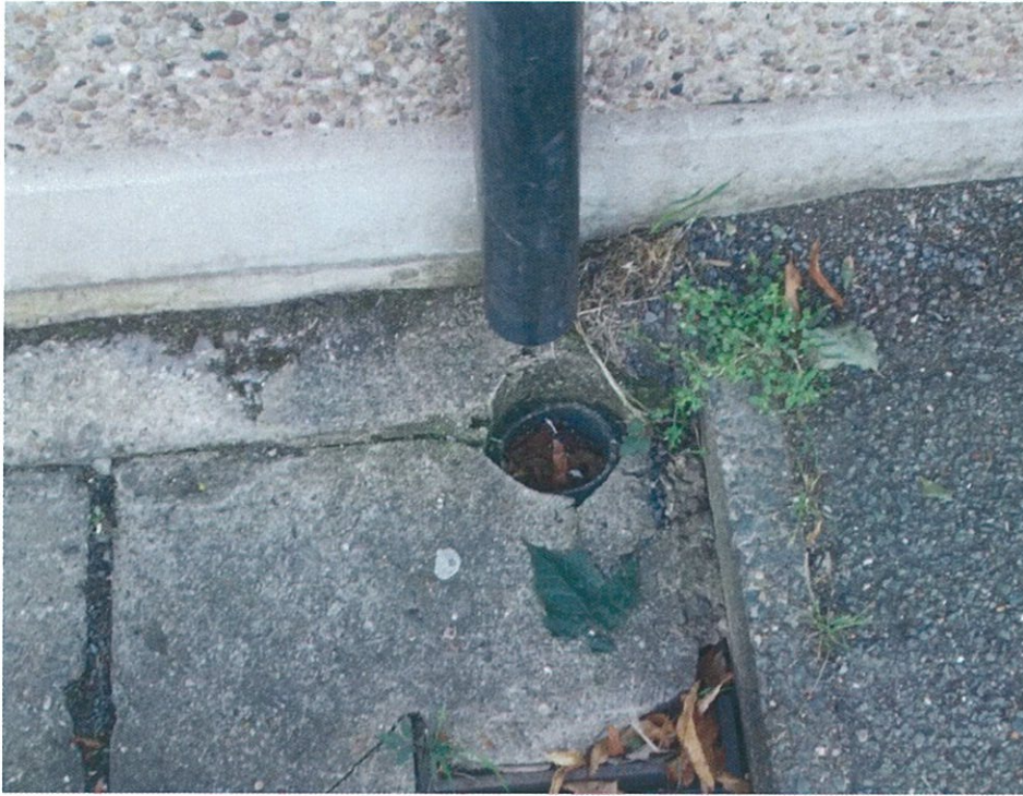
Photo 9 Example of Broken Downpipe
